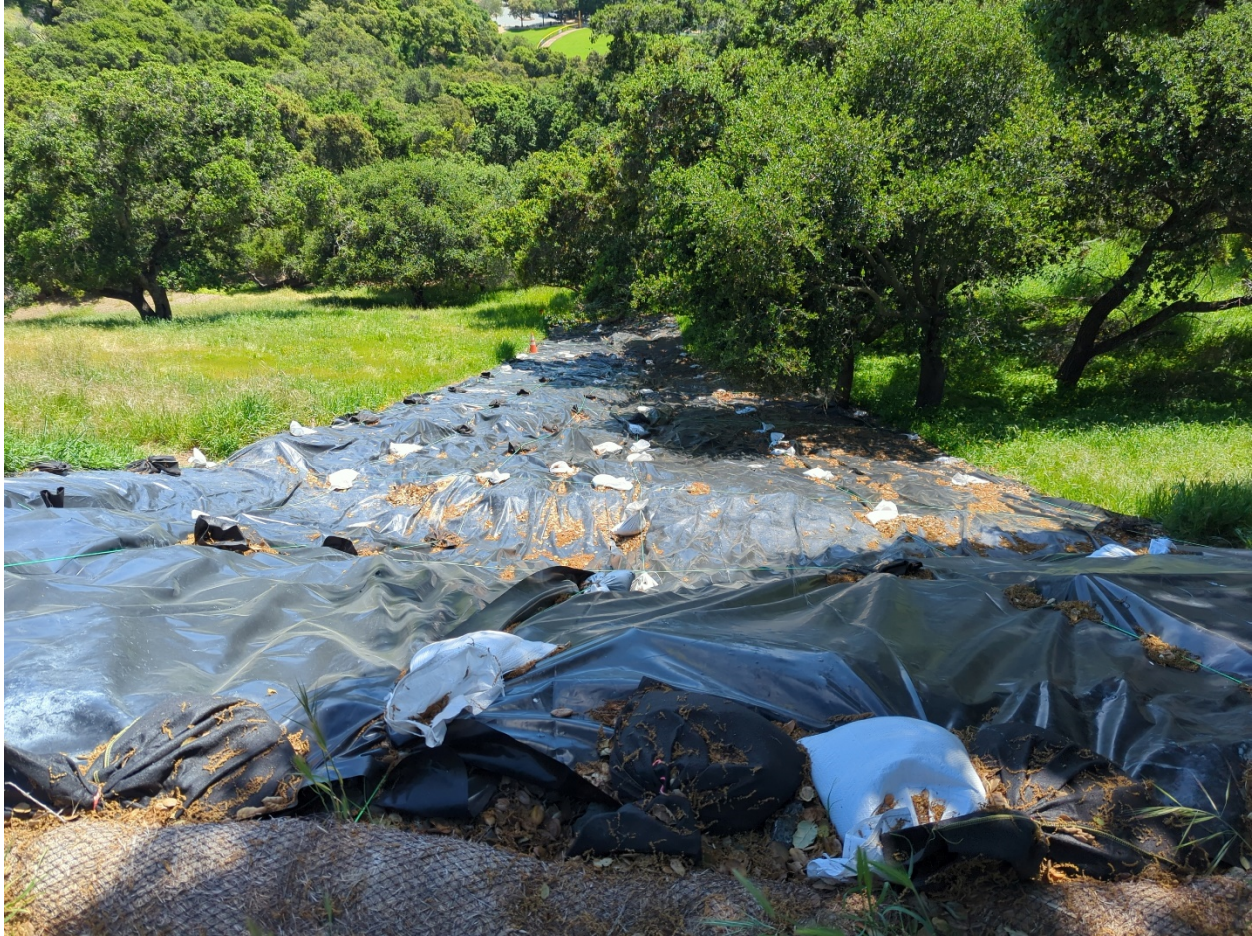
Exhibit 2. Temporarily stabilized landslide from the 2022-2023 storms along Dartmouth Ave above Arguello Park. Photo taken by WRA 4/12/24.
