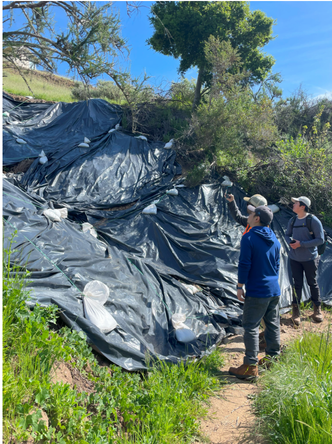
Representative example of recent landslide and treatment at Big Canyon Park.
