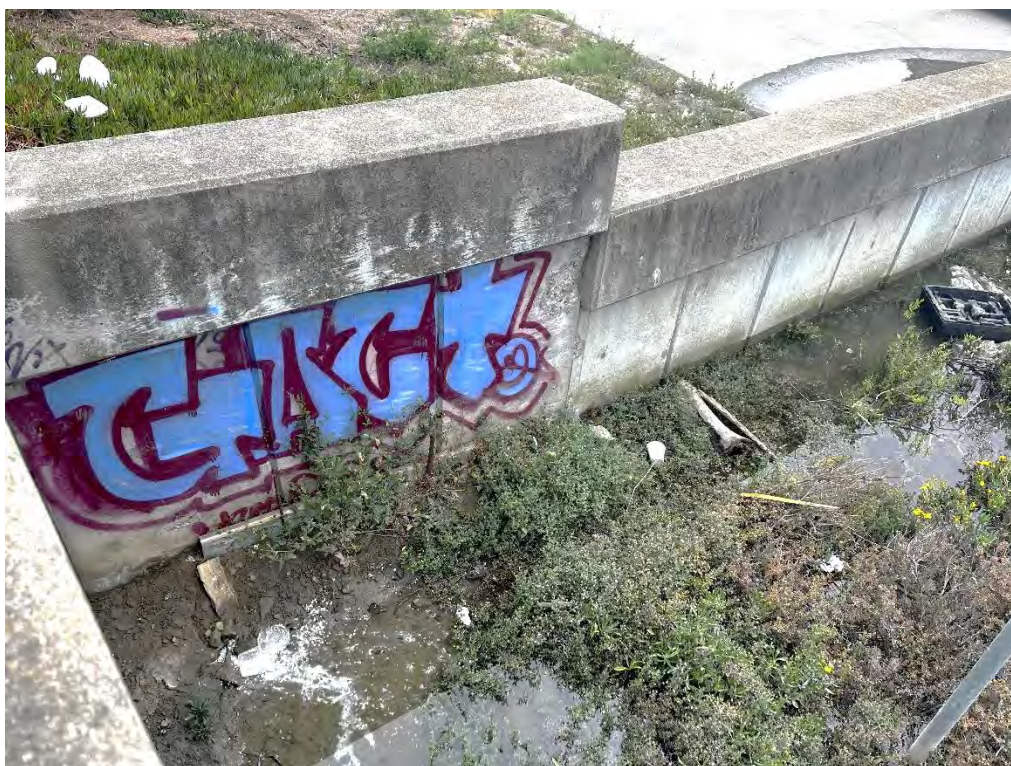
Photos 5 & 6 — Top photo shows erosion under the wing wall at the northwest corner of Utah Avenue. Bottom photo shows the wing wall at the northeast corner of Utah Avenue. Graffiti and trash from sources including upstream drains and illegal dumping noted along this reach.
