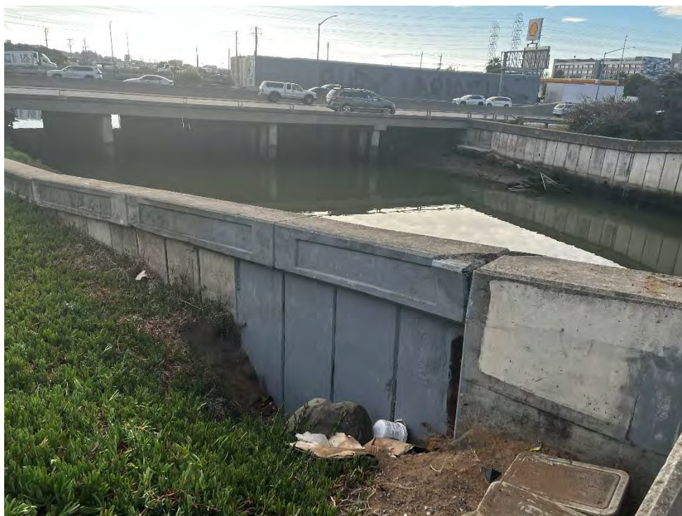
Photos 13 & 14 — Top photo shows damage on channel wall and partially blocked culvert outfall downstream from the Produce Avenue bridge facing the Highway 101 crossing. Bottom photo shows void outside the channel well. Trash dumping continues to be a challenge in these reaches.
