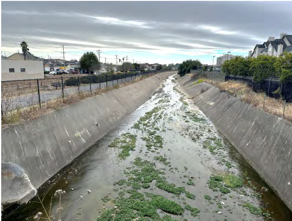
Photos 29 & 30 — Top photo shows culvert obstruction at Centennial Way. Bottom photo shows Colma Creek looking downstream from the BART culvert.
